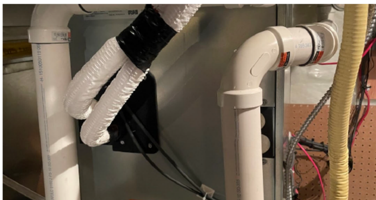
Heat pump indoor unit
