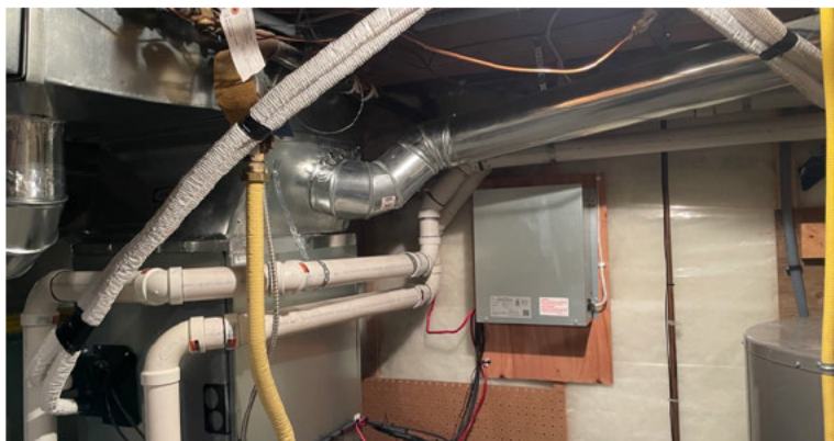
Heat pump indoor unit2
