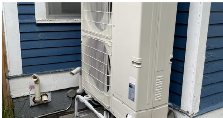
Heat pump outdoor unit
