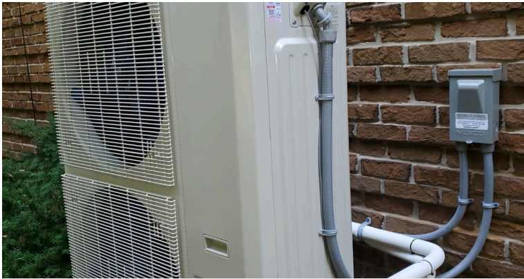
The new air source heat pump
