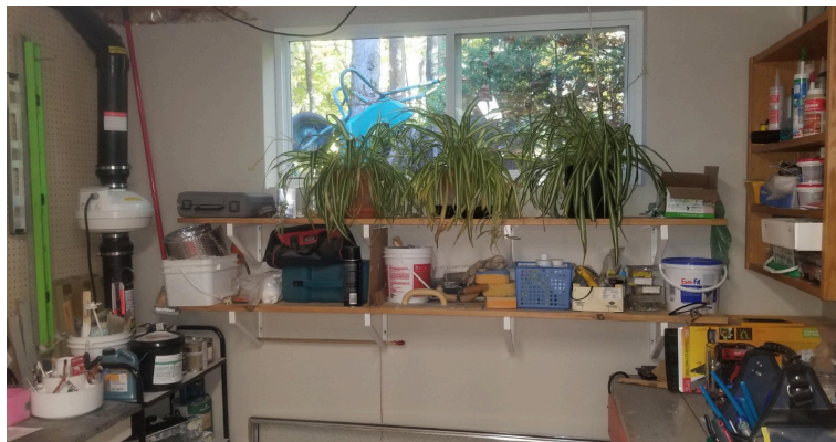
Customer already had soil gas extraction fan.
