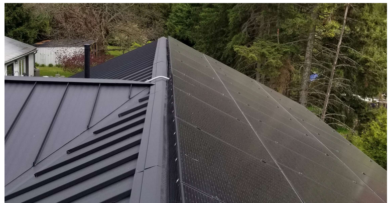
Solar on roof
