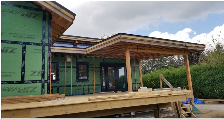
ZIP system panels used
