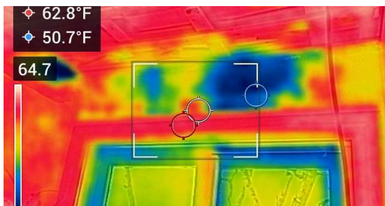
Thermal imaging at doors
