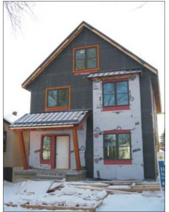
■ MILL CREEK Net Zero home in Edmonton is a second project being built by the team that produced the Riverdale Net Zero house — at a 40% lower cost because of what was learned on the first project.
